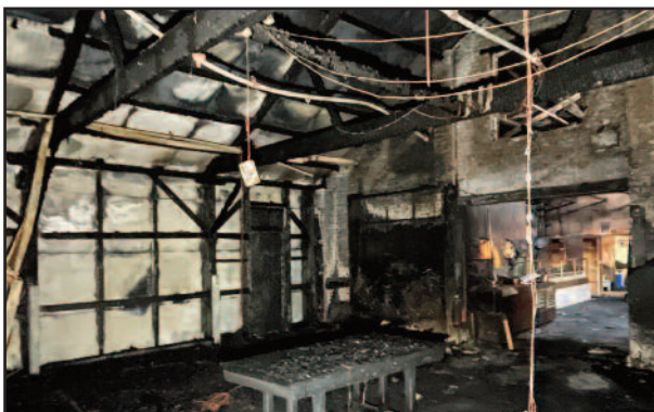
2022 fire damage to cafe and gallery
